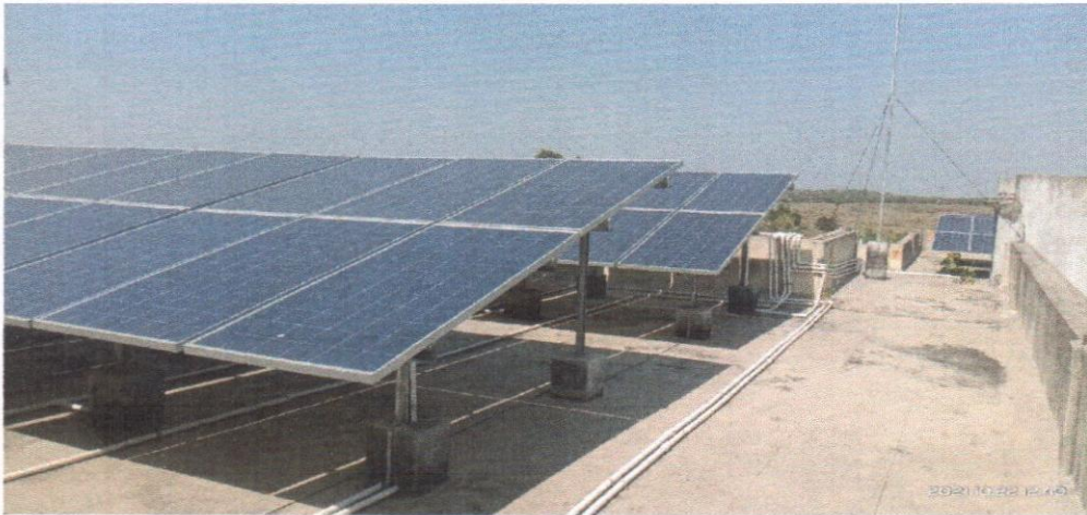
300 kW Roof top Solar system at Dr.VithalraoVikhePatil Foundation (Engineering, IBMRD, Junior, Agri College Feeder)
